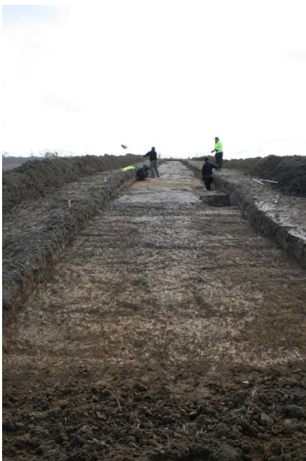
Left: 2015: As one local said, 'Are you archaeologists? Or are you laying a gas pipe?'
